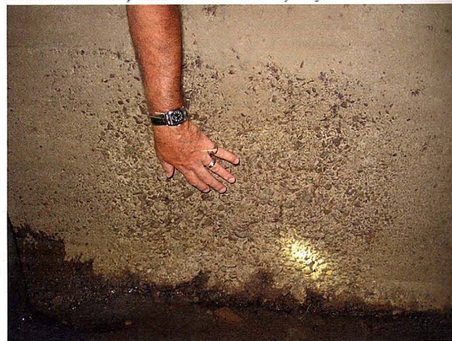
Deterioration included surface spalling, joint deterioration, wall blowouts and vertical wall cracks.
