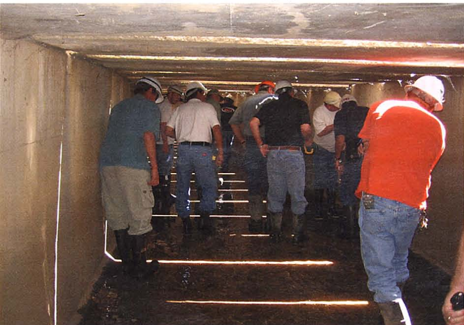
The project team inspected the flume to determine the scope of work required.
