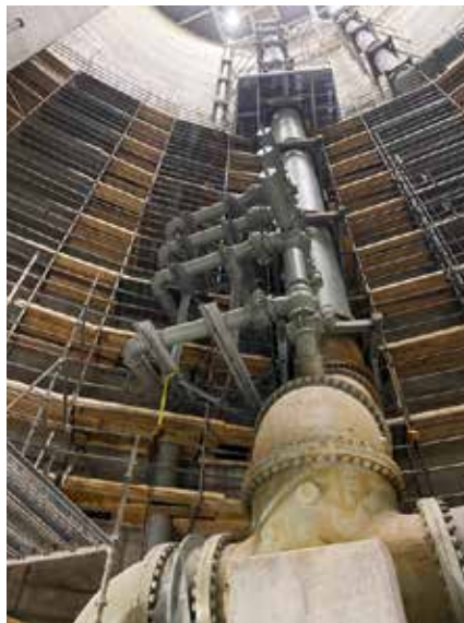
Fig 5 -- More than 7,600 pieces of scaffolding were required to reach the circular walls lining of the lift station in order to apply several Xypex products to repair and protect the concrete. Other corrective measures taken included replacing badly corroded steel pipe with stainless steel pipe and steel ducts and plenums with fiberglass.
