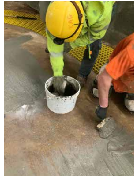
Fig 9 -- The lift station floor was coated with Xypex Concentrate and Megamix I fortified with Xycrylic Admix.
