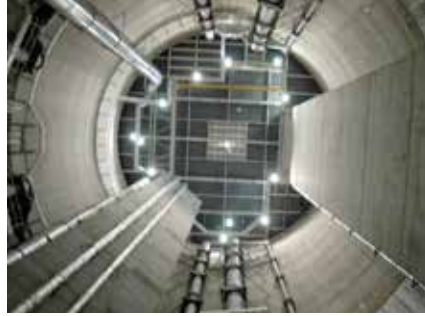
Fig 4 -- Looking up from 223 feet below ground to the top of the lift station. Ground water intrusion and constant high humidity led to serious corrosion and deterioration within just a few years.
