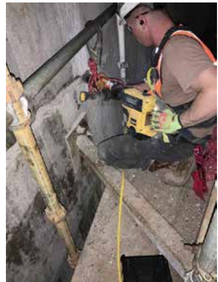
Fig 6 -- More than 3,100 feet of joints and cracks were jackhammered, cleaned and plugged before the walls were sealed with a Xypex Concentrate, Modified and Gamma Cure.
