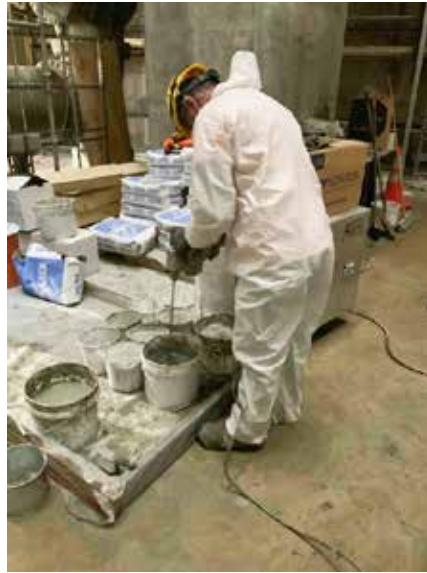
Fig 8 -- Xypex Concentrate is premixed for brush application to the lift station walls. Concentrate in Dry-Pak form was used to fill construction joints and cracks. Actively leaking cracks were filled with Xypex Patch'n Plug.
