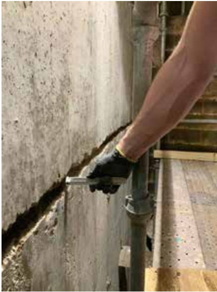
Fig 7 -- All cracks and joints were jackhammered, cleaned and plugged. Here, an applicator checks the readiness of a long crack.
