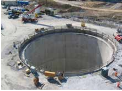
Fig 3 -- During construction of the 223 ft deep by 90 ft in diameter lift station shaft. Slurry wall construction was used to reach bedrock at about 100 feet.
