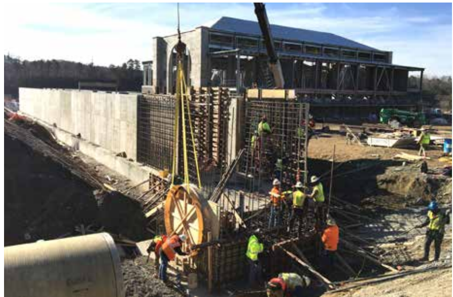
Fig 9 – Elaborate form work and reinforcement was needed to integrate multiple large pipes into the concrete channel at both the Bellwood Quarry and Hemphill pumping stations.
