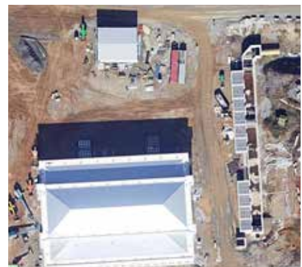
Fig 6 – Overhead view of the Bellwood Quarry pumping station under construction. The concrete flow control channel (at right above) was cast in place with Xypex Admix C-500 as part of the 5,000 psi mix. Xypex Admix provides integral waterproofing and protection that will help the structure meet its 100-year design goal.
