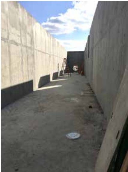
Fig 7 – A look inside the flow control channel at the Bellwood Quarry pumping station. More than 1,000 cubic yards of 5,000 psi concrete was treated with Xypex Admix C-500 crystalline waterproofing.
