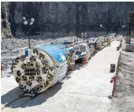
Fig 2 – The 400-foot long TBM dubbed “Driller Mike” is readied for launch on the floor of the Bellwood Quarry in September 2016. The TBM would be used to drill a 12.5-foot diameter tunnel through five miles of solid rock from the quarry to the Chattahoochee River.
