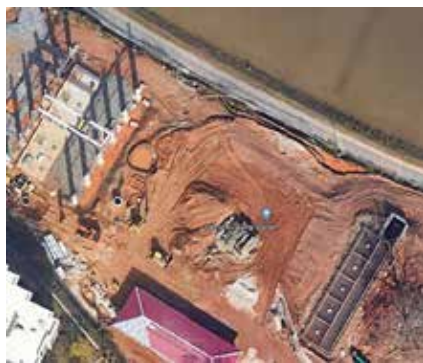
Fig 5 – Overhead view of Hemphill pumping station under construction. Cast-in-place concrete channel is at lower right.
