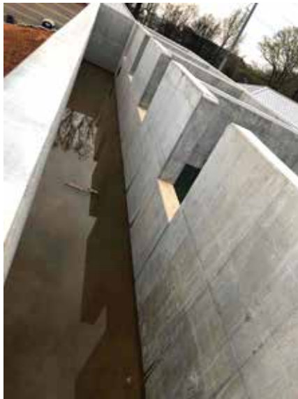
Fig 8 – Hemphill pumping station flow control channel was cast in place with Xypex Admix C-500 as an integral part of the mix.
