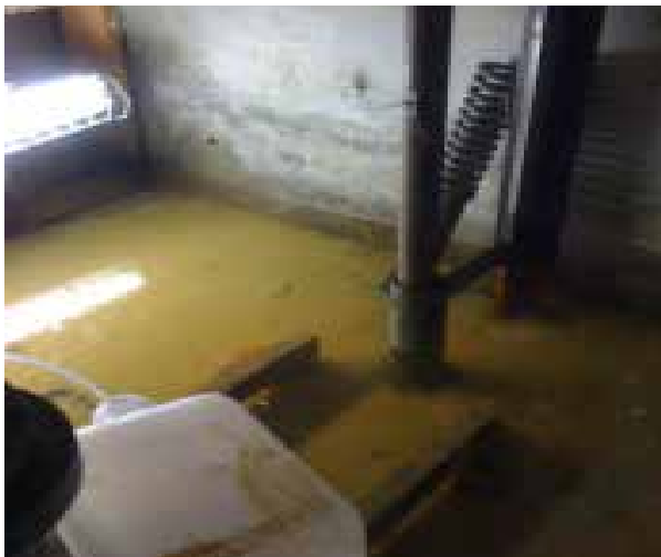
Water Ingress in Elevator Pit
