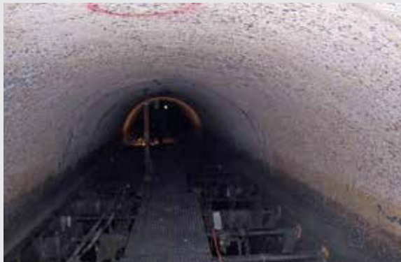
Inside of pipe pressure-washed in first 8-hour closure. Note the very rough surface with exposed aggregate caused by cement paste loss.
